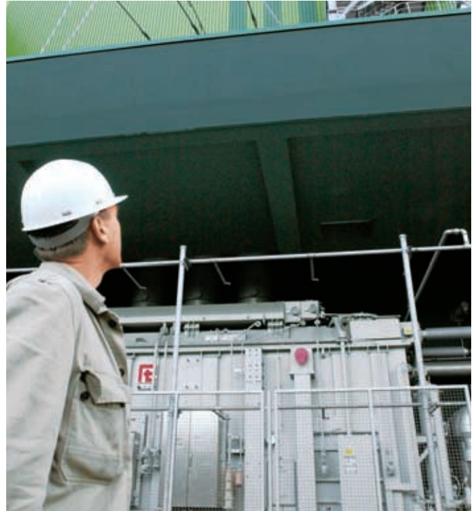
Powerhouse | This transformer, manufactured by Belgian company Pauwels, at the Duisburg-Hamborn power station transforms 332 MVA (megavolt-amperes) of power - enough to supply a medium-sized city. Photos: Rainer Schröder
